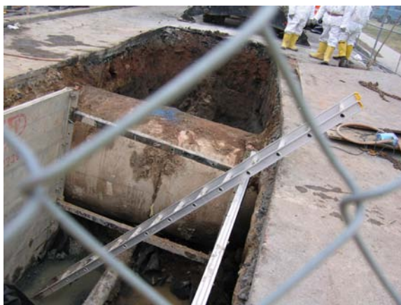
View of full excavation of damaged water line; repairs were performed by the Passaic Valley Water Company.
