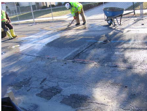
View showing initial conditions of the pavement on Columbia Lane.
